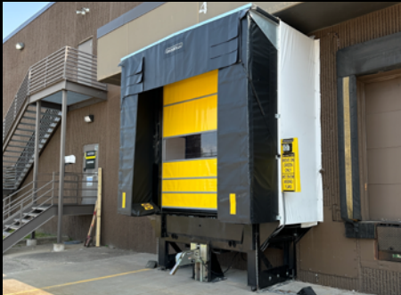
EXTERIOR DOCK LEVELERS
